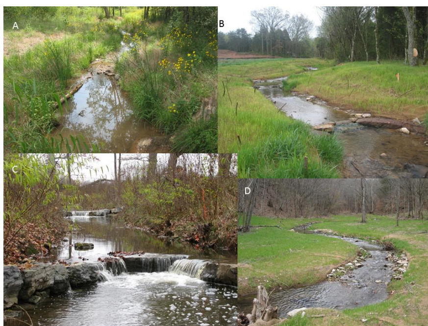
Figure 4. Structures used for stream restoration. A. A small log vane is used to stabilize the bank immediately upstream of a small constructed riffle. B. Cross-vanes are used for bed stabilization. Newly planted willow stakes line the bank and constructed mini-floodplain. C. Cross-vanes and established willow stakes. D. Root-wads, constructed riffles, and artificial meanders.
