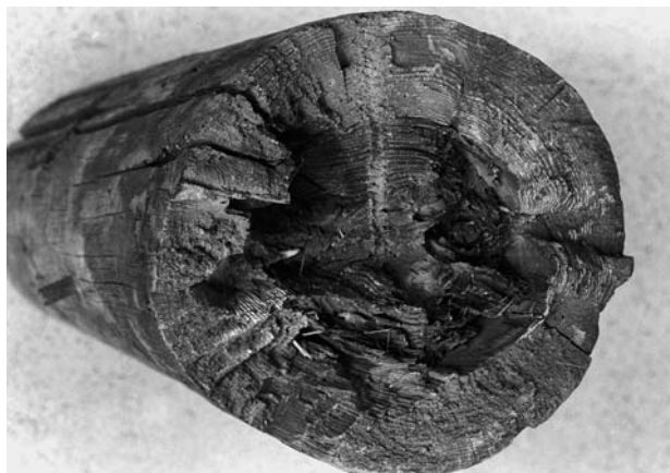
Figure 10.16. Severe soft rot attack in a preservative treated transmission pole has resulted in a brash fracture.
