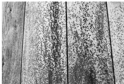
Figure 10.21. Heavy mould growth on untreated oak wood panels.
