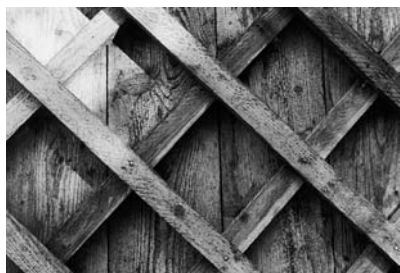
Figure 10.22. Mould growth on untreated larch wood panels and battens.
